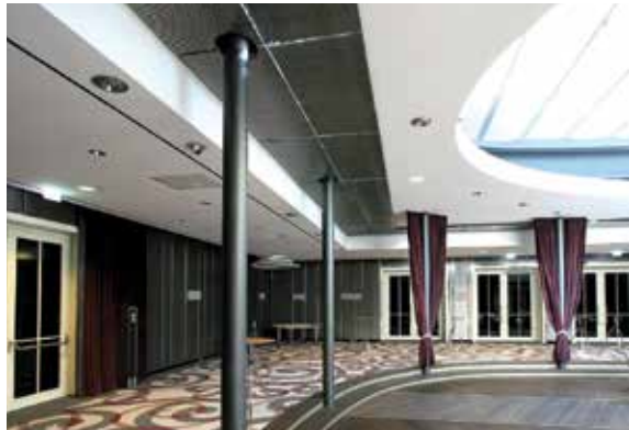
Chilled ceiling, Hotel Steigenberger Drei Mohren, Augsburg, Germany Architect: Alpstein | Mesh: Atlantic (4)
